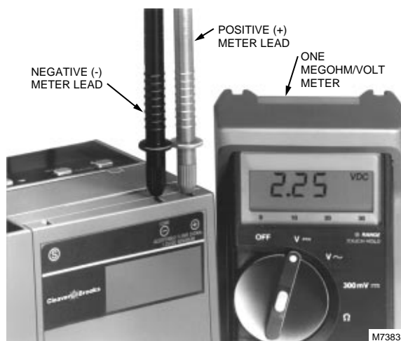
Fig. 22. Flame signal measurement.
