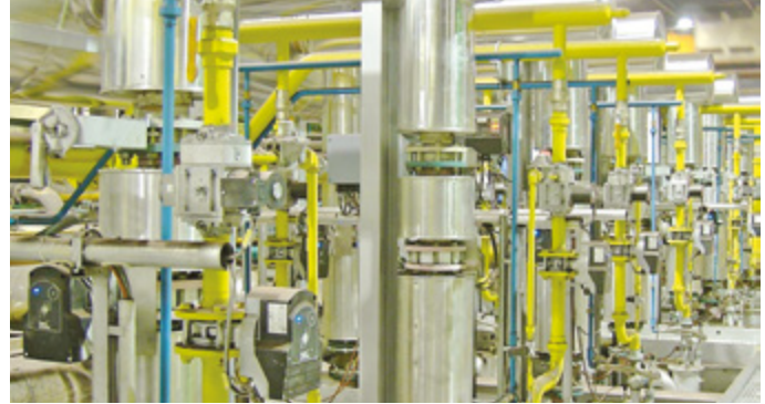
Walking beam furnace with overhead firing
