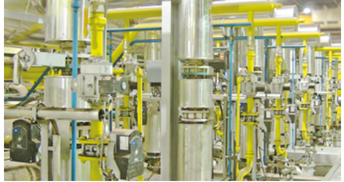
Walking beam furnace with overhead firing
