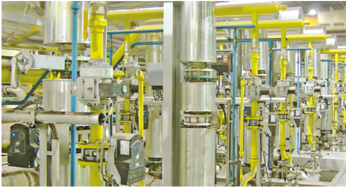
Walking beam furnace with overhead firing
