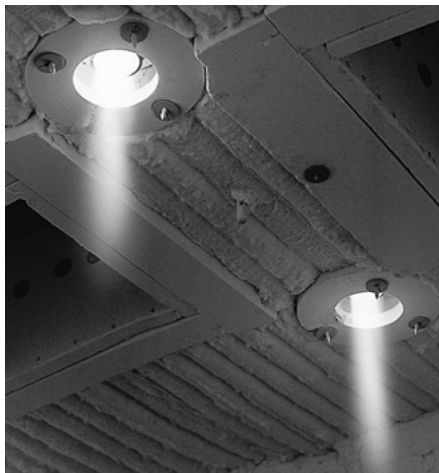
Overhead heating with burner BIC
