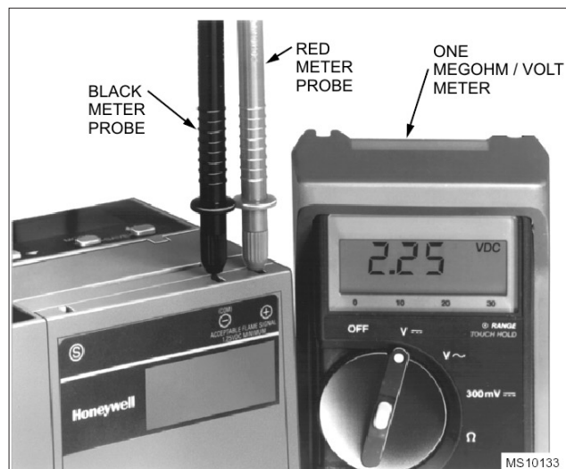
Fig. 11. Measuring voltage flame Signal with 7800 SERIES controls
